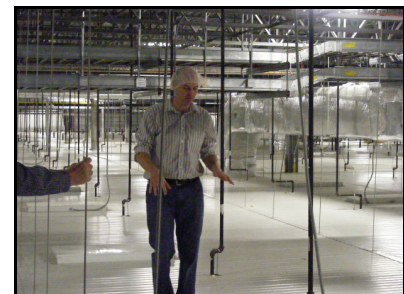
▲ Jarrod Sharpe, Kitchen Facility Manager, explains the construction and capabilities of “walk-on” ceiling.
