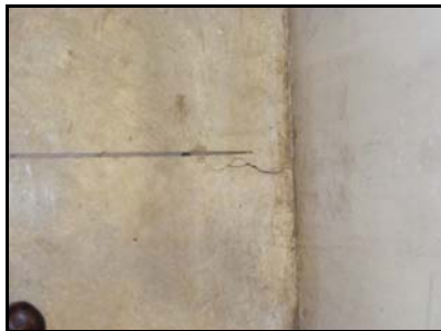
▲ Cracking resulting from shallow sawcut control joint stopping short of wall
